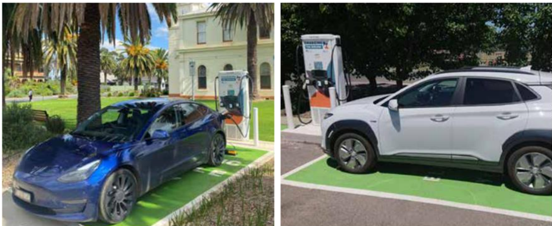
Electric charging stations at Inglewood and Wedderburn.
