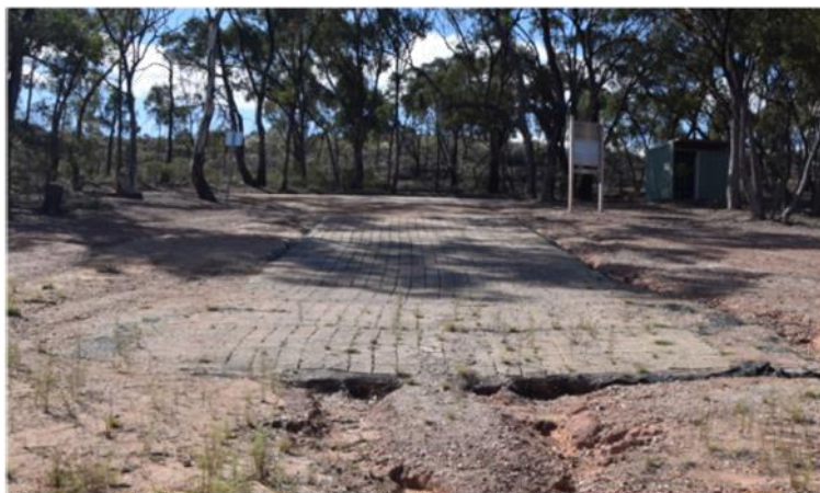
Figure 7.3 Existing boat ramp cracking and erosion.
