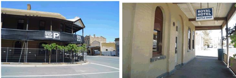
The Verdon Street single storey section is in relatively, good condition as too the facade along Brooke Street. The verandah along Brooke Street is in better condition than the two-storey section in Verdon Street. However, the corrugated balustrade is inappropriate and the dead weight loading too heavy for the structure.
