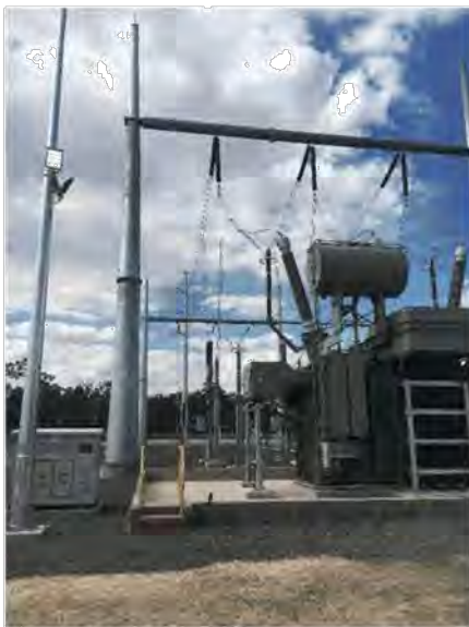
Example of substation
