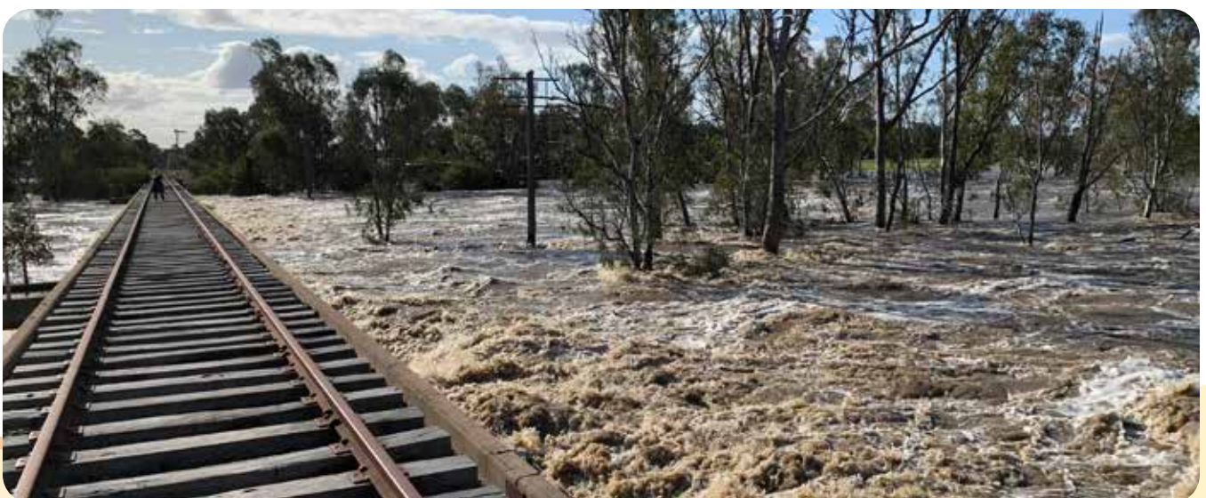
Top: Bridgewater floods. Above: Railway track crossing the Loddon River at Bridgewater-on-Loddon.
