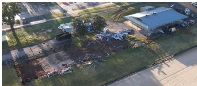
Demolition works took place in August for the Donaldson Park Community Hub project.
