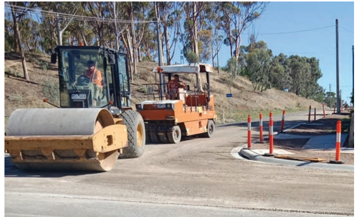
Works taking place at Lake View and Andrews Street in Boort, which are now complete.
