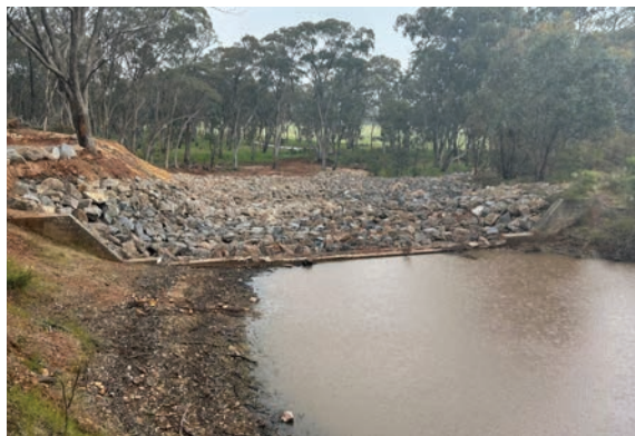
Emergency works at Skidders Flat Reservoir spillway included widening of the spillway and installation of an additional 1600 tonnes in total of rock beaching.
